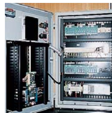
Top: Fuel gas compressor, Mitsubishi Motors, Japan Above: Compressor control panel Below: Varanus Island
